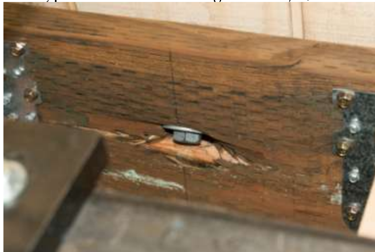
Figure B12. Typical Failure for Configuration 4, 5/8-inch Lag Screw
