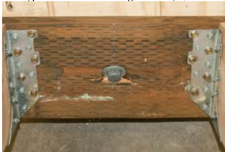
Figure B14. Typical Failure for Configuration 4, 5/8-inch Lag Screw
